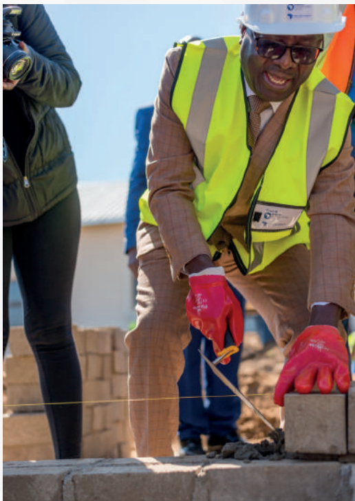
The Honourable Minister of Urban and Rural Development for Namibia lays a foundation stone during the NIC Launch on 27TH April 2021
